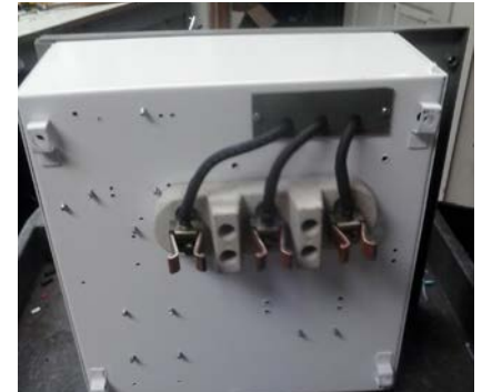
Stabs installed on unit
